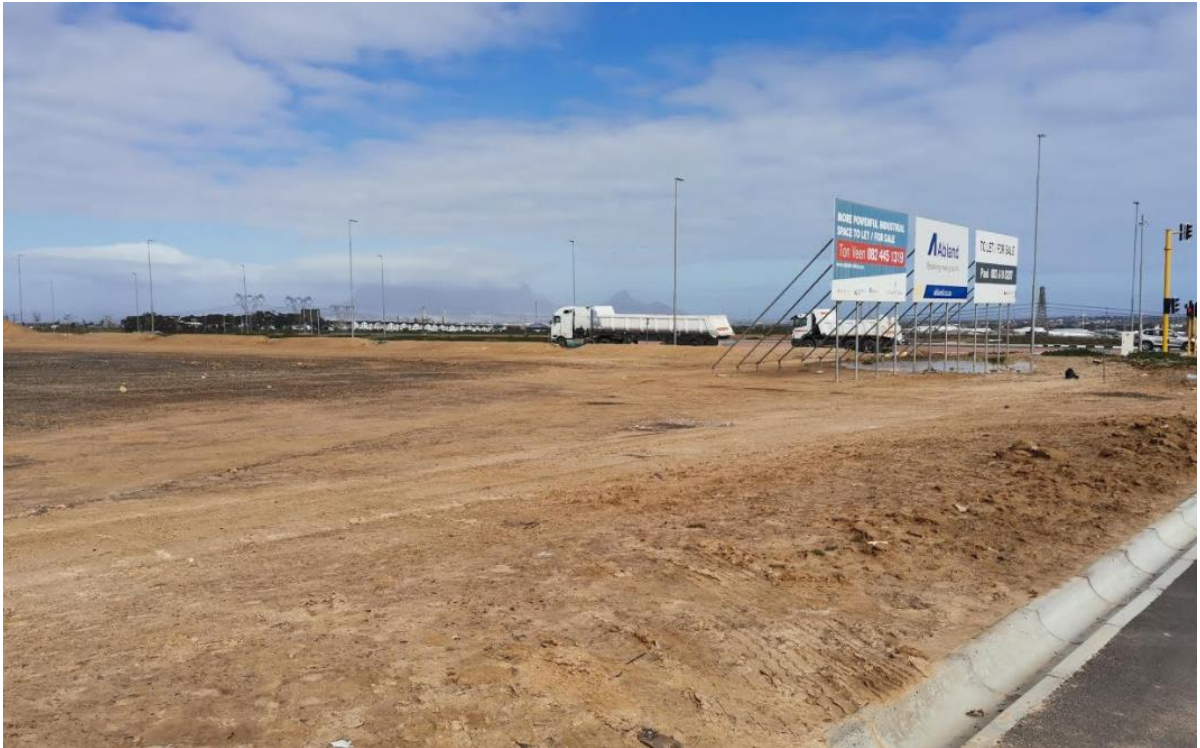
Photo 2: The site has been cleared and grubbed, with development platforms completed in preparation for development.
