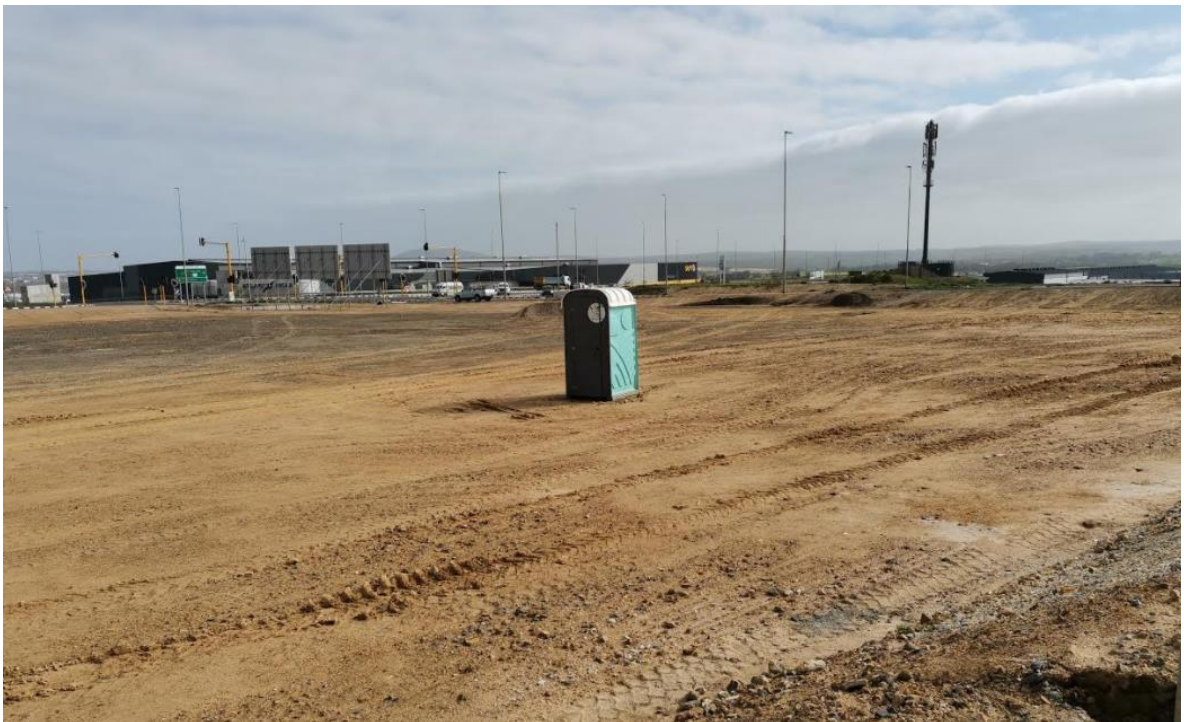
Photo 3: View over the site towards the intersection between Giel Basson Drive and Welbeloond Road
